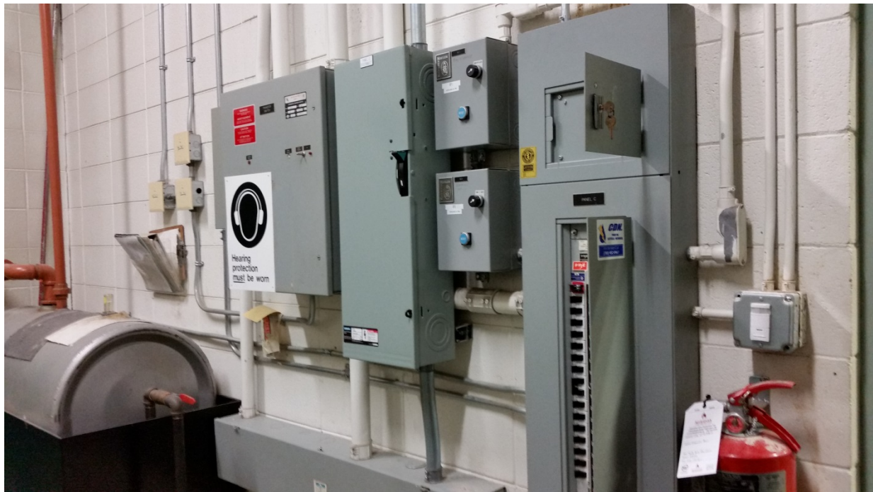
Photo 5 – Sub Distribution Panels and Motor Controls
