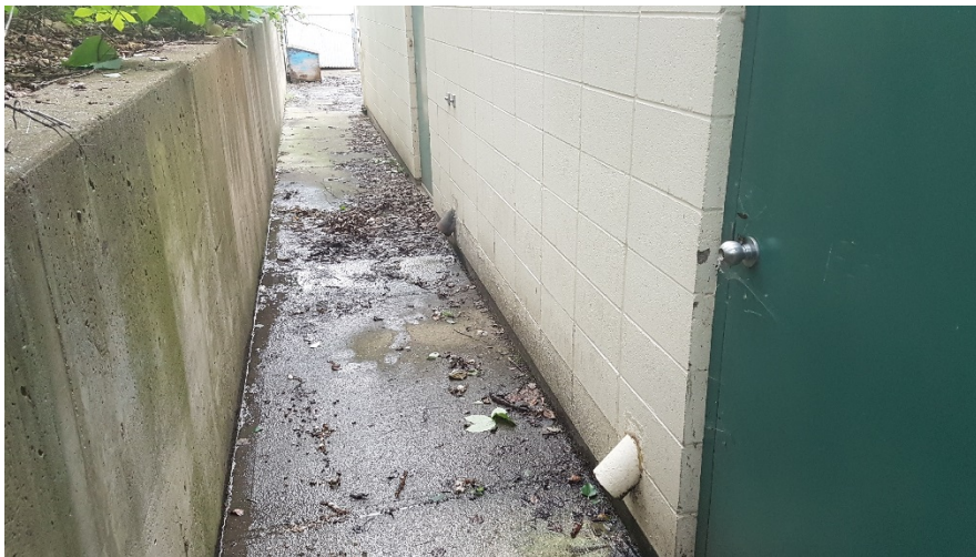
Photo 6 – Roof drains splashing to grade
