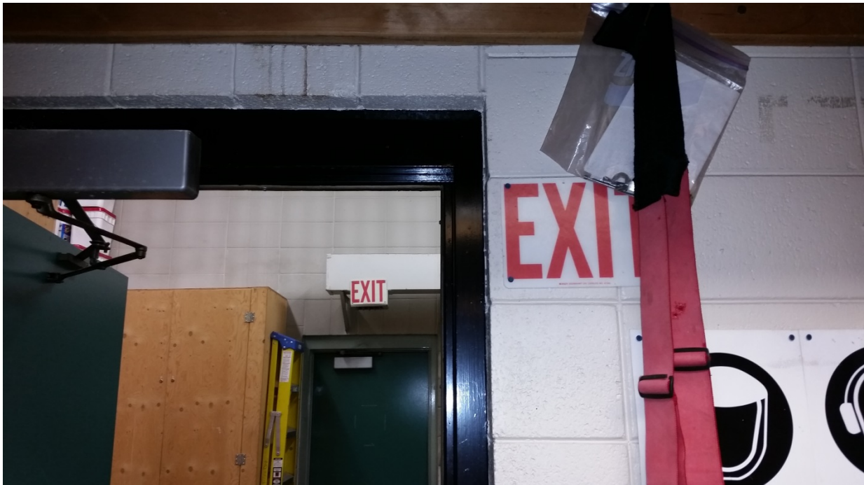
Photo 23 – Paper Exit Signs
