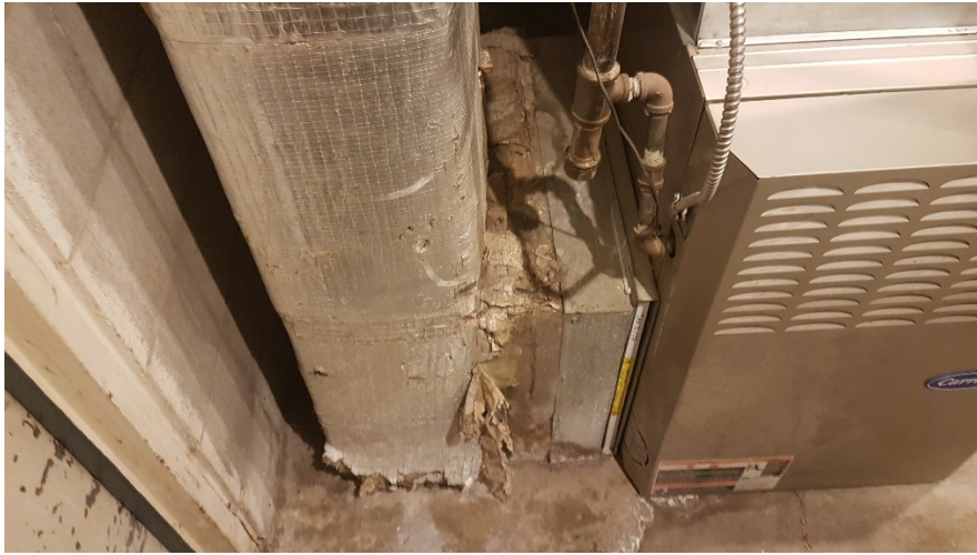
Photo 5 – Damaged duct insulation
