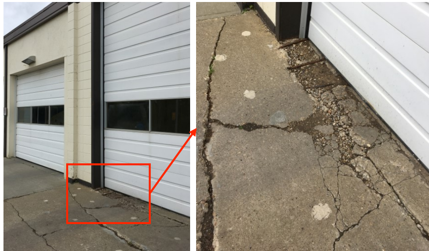
Photos 7 and 8: Apron slab deterioration at west overhead door
