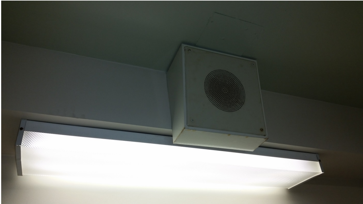
Photo 21 – Old Rusted Speaker
