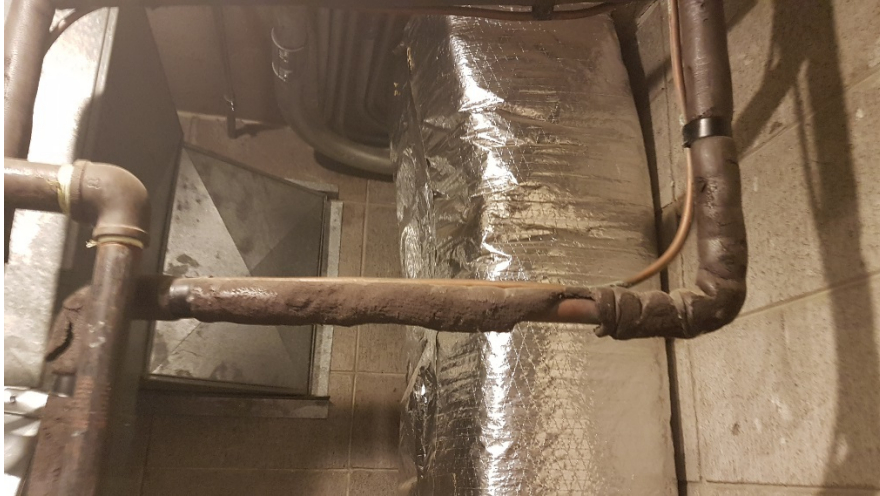
Photo 4 – Damaged refrigerant pipe insulation
