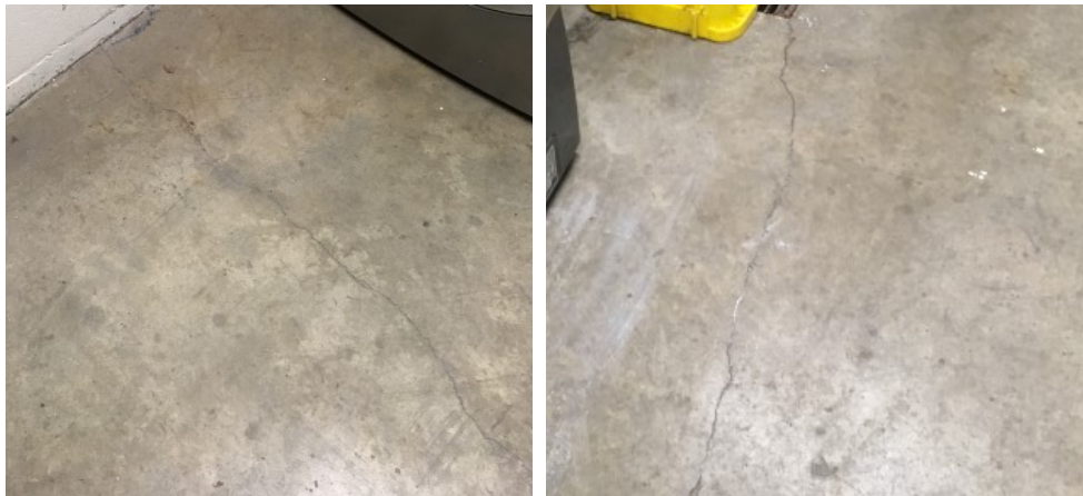
Photos 5 and 6: Typical cracks in slab-on-grade
