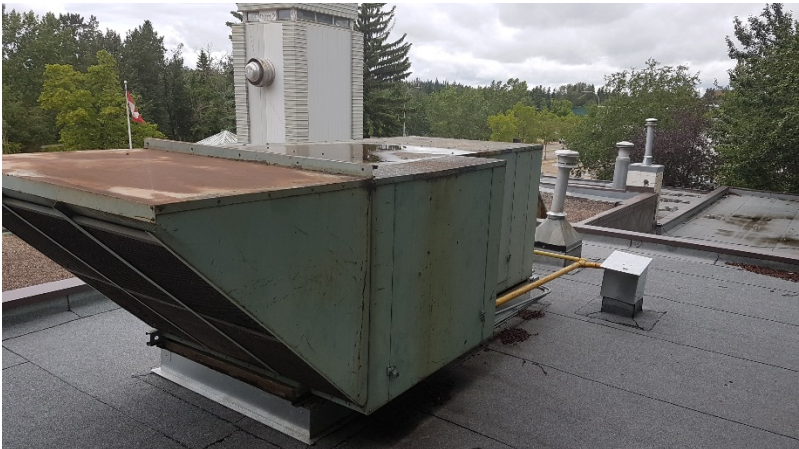
Photo 1 - Apparatus Bay Makeup Air Unit
