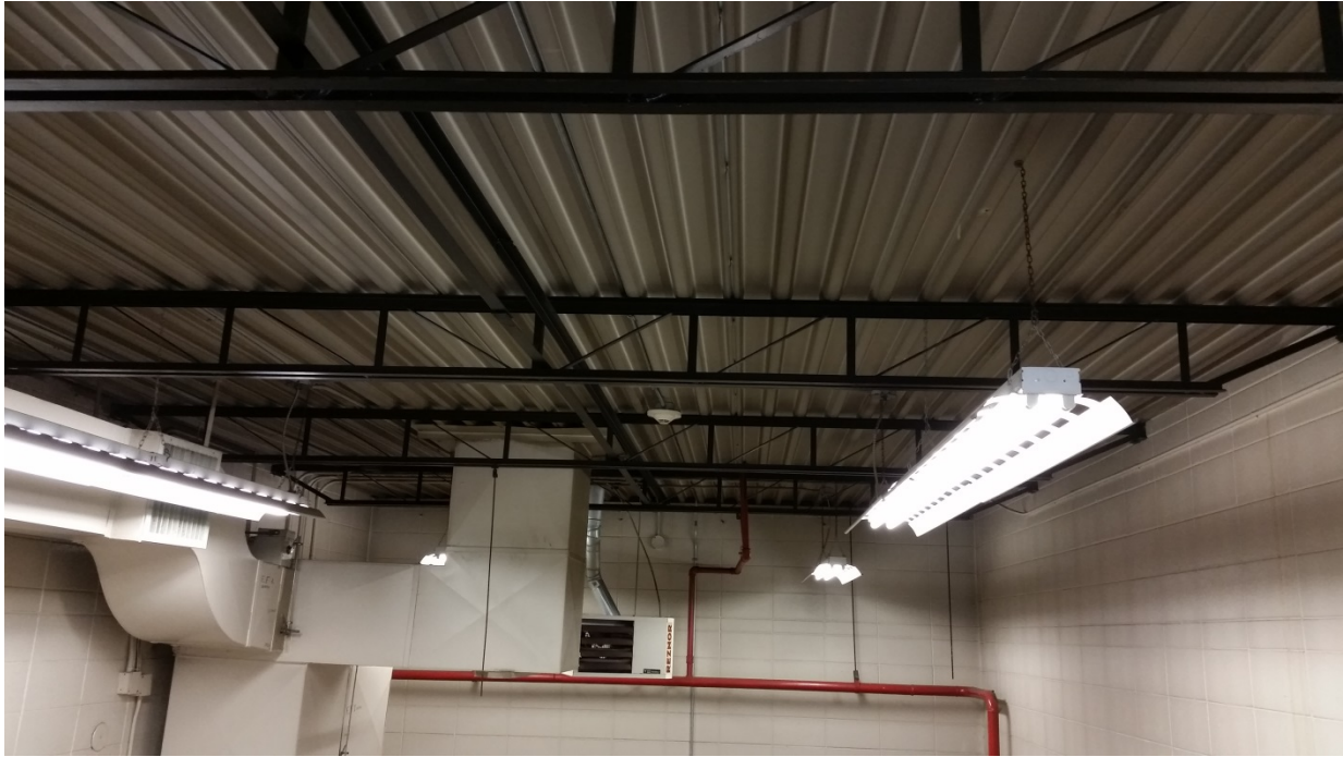
Photo 14 – Apparatus Bay Lighting
