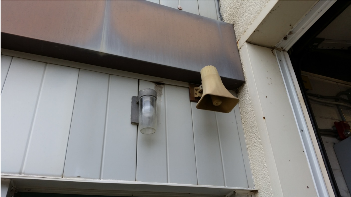
Photo 9 – Exterior Incandescent Fixture and Speaker
