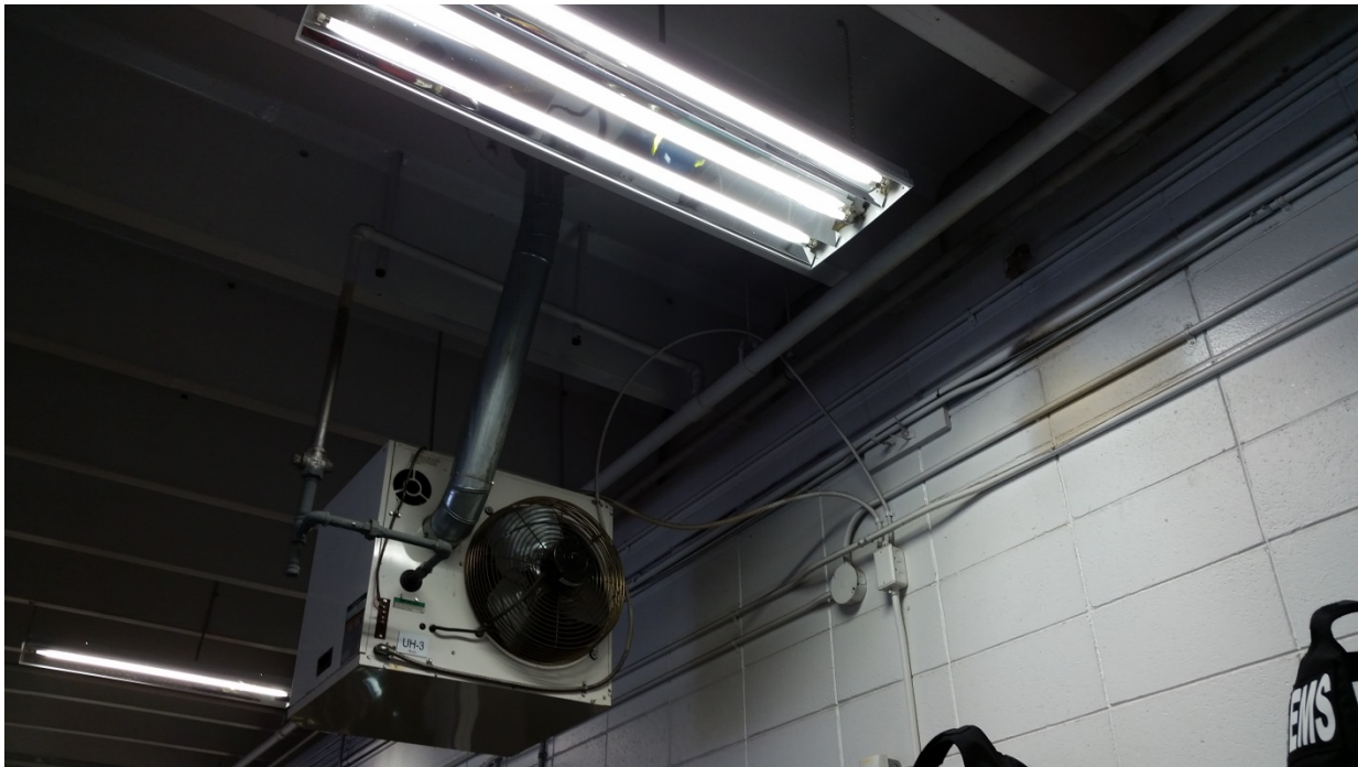
Photo 15 – Gear Room Lighting
