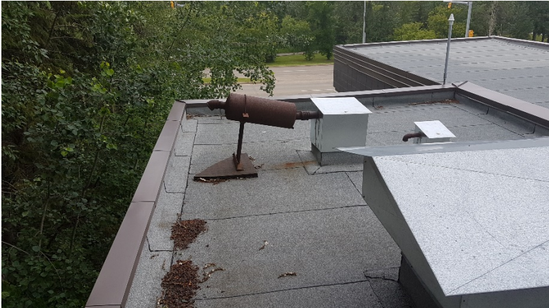
Photo 2 – Emergency Generator Exhaust Muffler
