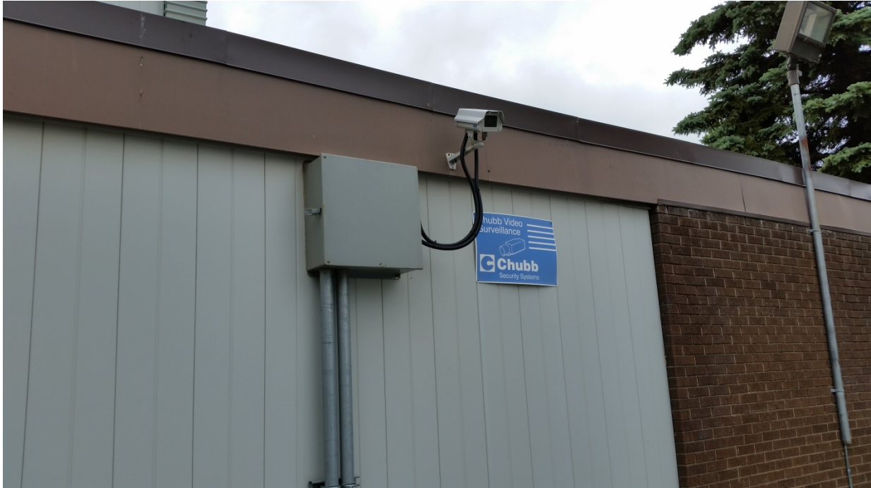
Photo 11 – Exterior HPS Fixture and Security Camera
