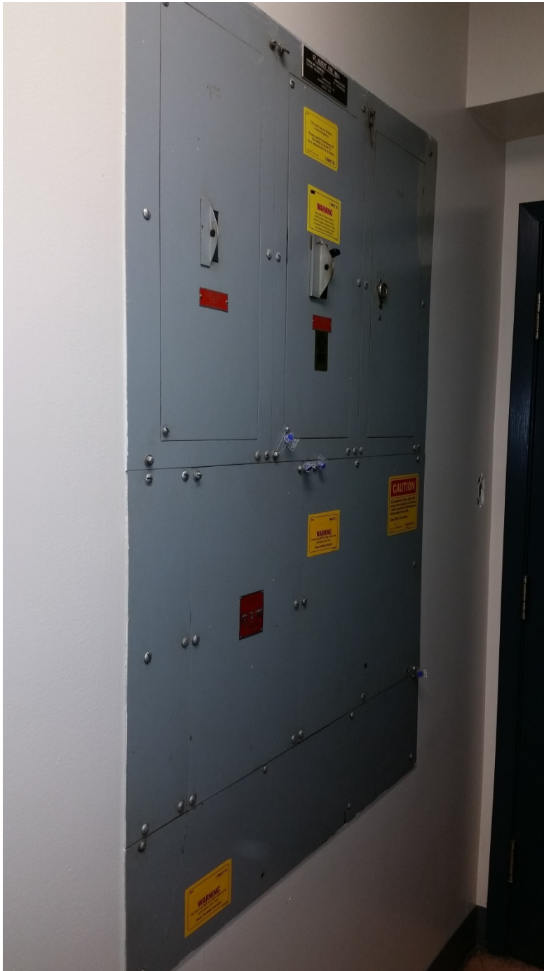
Photo 1 – Main Service Distribution
