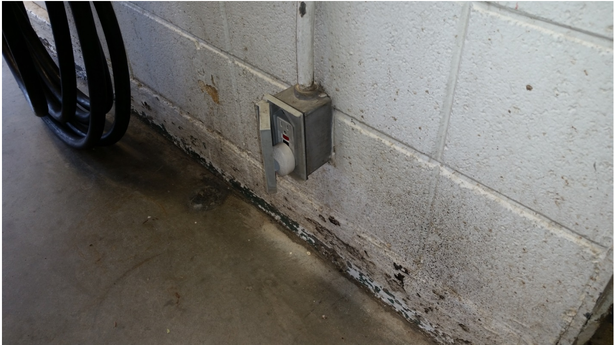
Photo 7 – Apparatus Bay Receptacle
