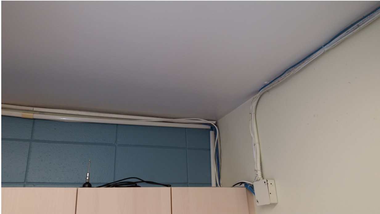
Photo 19 – Conduit Installation and Poorly Installed Data Cabling
