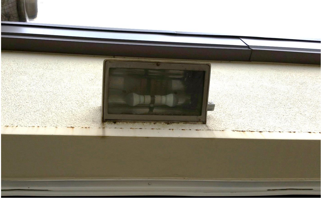
Photo 10 – Exterior Incandescent Fixture
