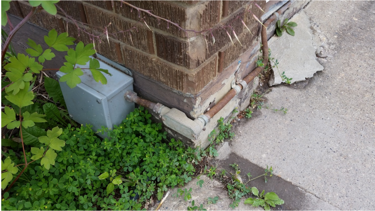
Photo 6 – Corroded exterior conduit
