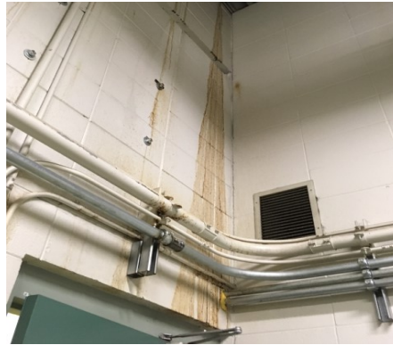
Photo 1: Roof leakage in generator room
