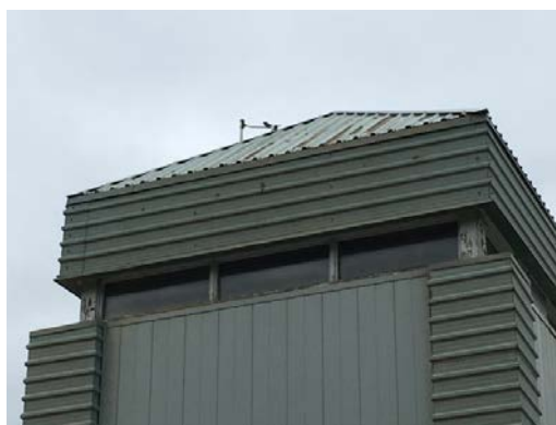
Photo 10: Deterioration of tower exterior finishes
